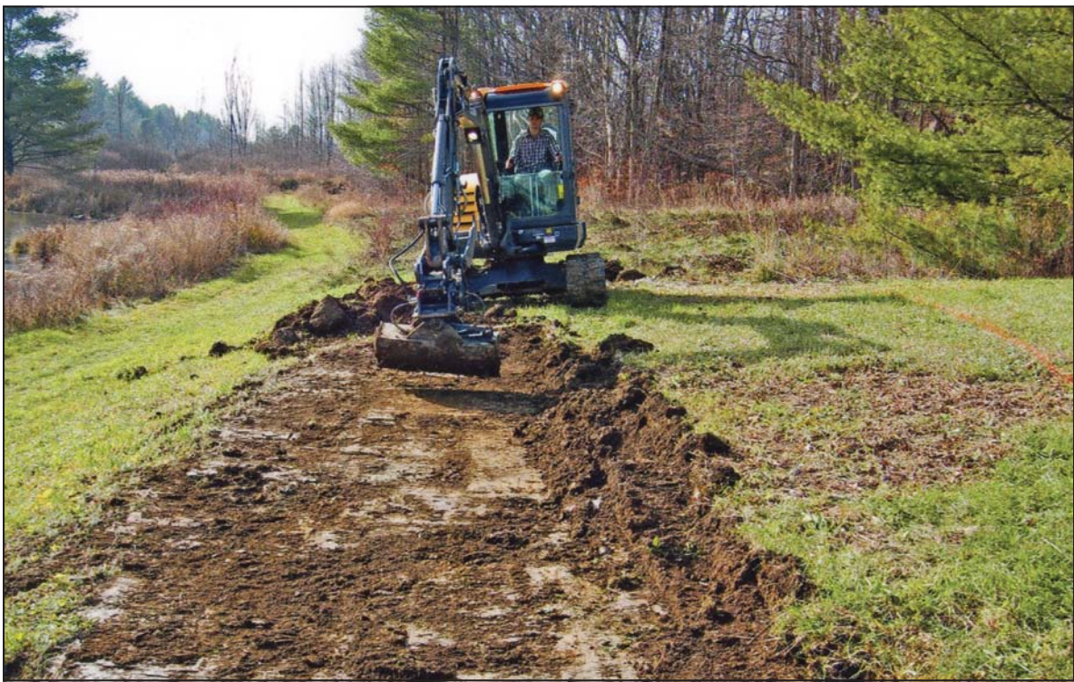
Work begins on the turtle nesting area, with a backhoe removing the surface vegetation. Photo by George Thompson
