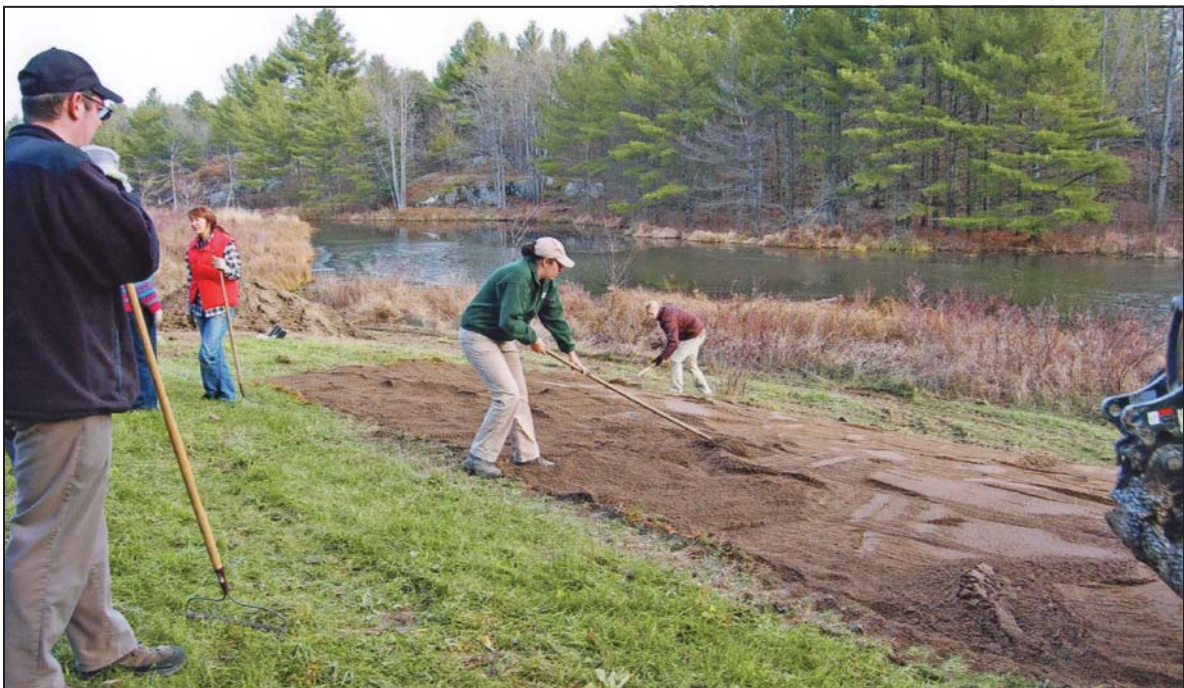
Finishing touches – a final layer of sand is spread over pea gravel. Having the beach so close to the water is critical, as is having it in a raised location so turtles can see it as they're swimming by. Photo by George Thompson
